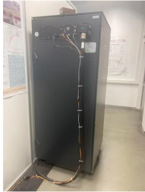
Figure 15. System's Generator Module
