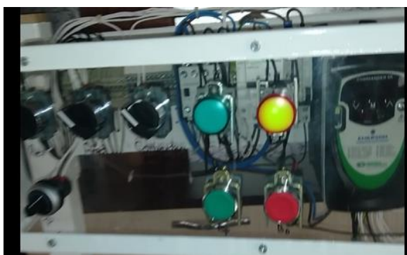
Figure 20. Light signaling: "No control voltage"
