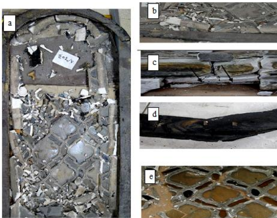
Figure. 1. The deterioration aspects of the stucco window number 454/7 in Cairo's Museum of Islamic Art
