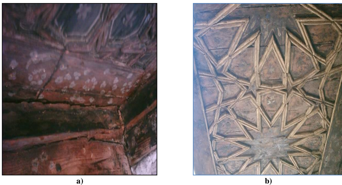
Figure 2. The ceiling of Abdel Rahman Katkhoda: a) staining of the ceiling with dusyt; b) decoration of the ceiling with geometric units.
