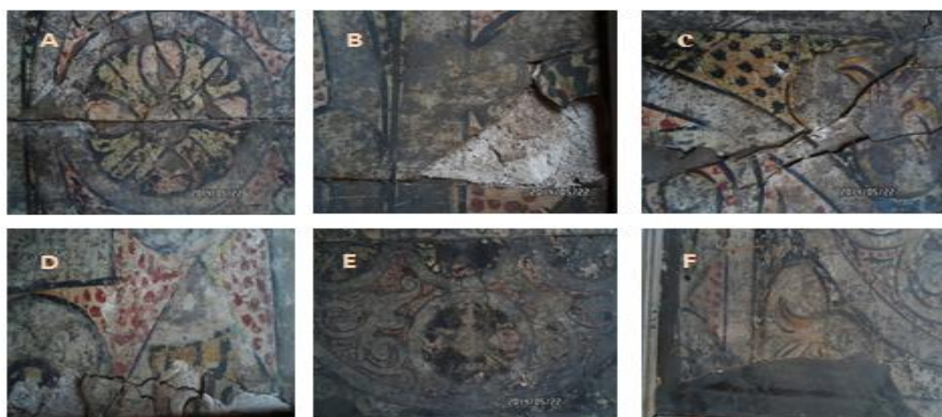
Figure 2. The condition assessment of the Coptic fresco painting: A - detachment in the body of painting; B - failure in paint layers; C - vital cracks; D - losses in painting layers; E - candle burns; F - resins materials from old conservation treatment.
